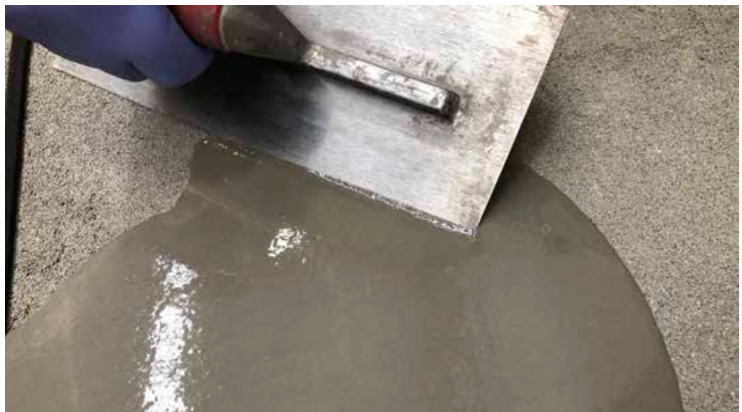
Installation of Ultraplan Trade after first priming the porous concrete substrate using Eco Prim T Plus diluted 1:2 with water
